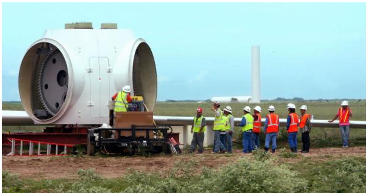
workers work connecting a blade to the rotator which goes on top of the towers to create a wind turbine. Workers are working feverishly now to ready more than 100 turbines before year is out or they loose their permit. This is at the Penascal Wind Farm south of Sarita. photo taken Tuesday. photo by George Gongora
