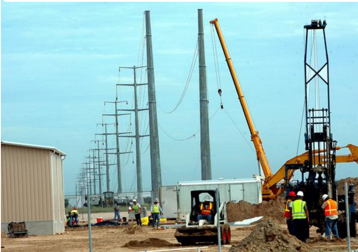
transmission lines from the Penascal Wind Farm south of Sarita are already being build. these lines will carry wind produced electricity. photo taken Tuesday. photo by George Gongora
